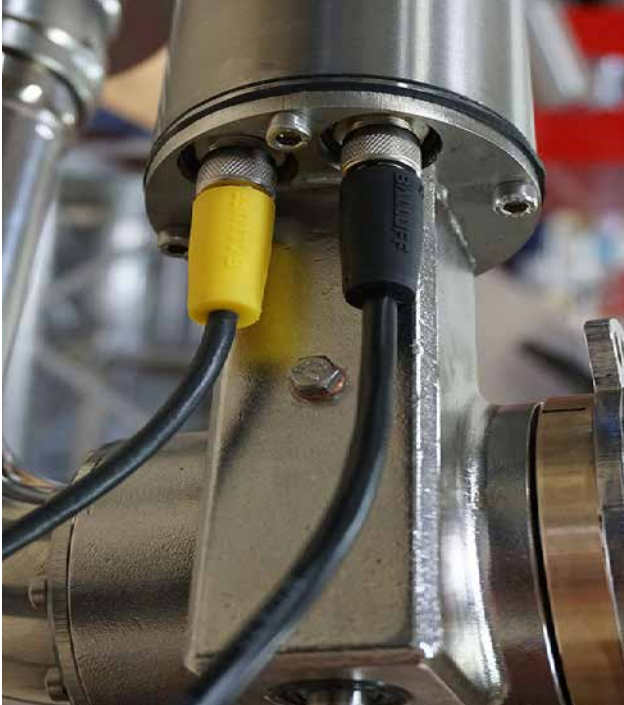
Phases and Sensor cable to vertical motor
